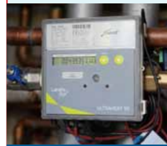
MONITORING HEAT DELIVERY AND SAVINGS
